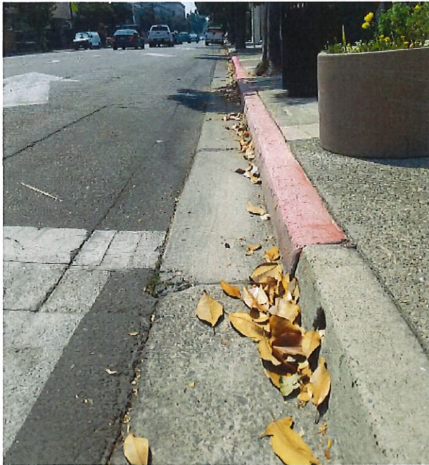
Gutter cleared at Red Inc Architects on J Street and 13 Street. (Before)
